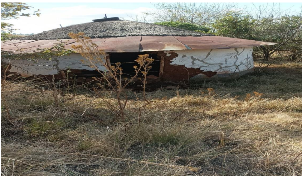
Figure 5.7: An abandoned house in KwaNokweja. (Source: Author, July 2022)
