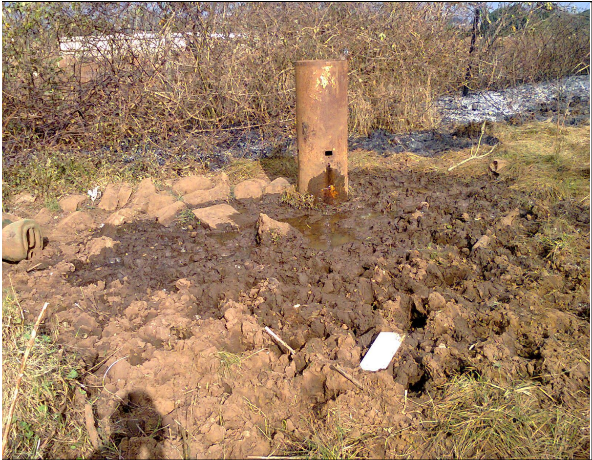
Figure 5:7 Some of the infrastructure used to provide water (Source: Researcher)
