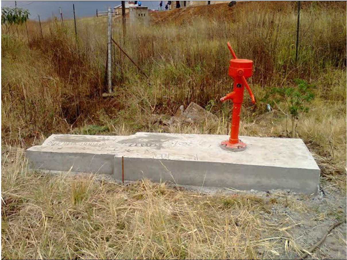
Figure 5:13 Borehole infrastructure in the Umzumbe Local Municipality
