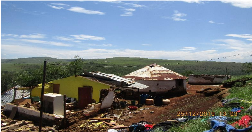
Figure 5.8: Mud houses affected by the tornado at uBuhlebezwe local municipality (source: Municipal Disaster Management Officer ubuhlebezwe local municipality, December 2019).
