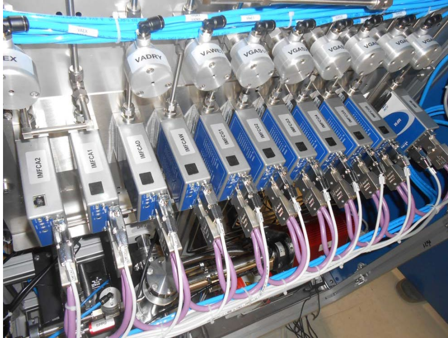
Figure 3.2.4.2: Gas distribution panel showing Mass Flow Controllers.
