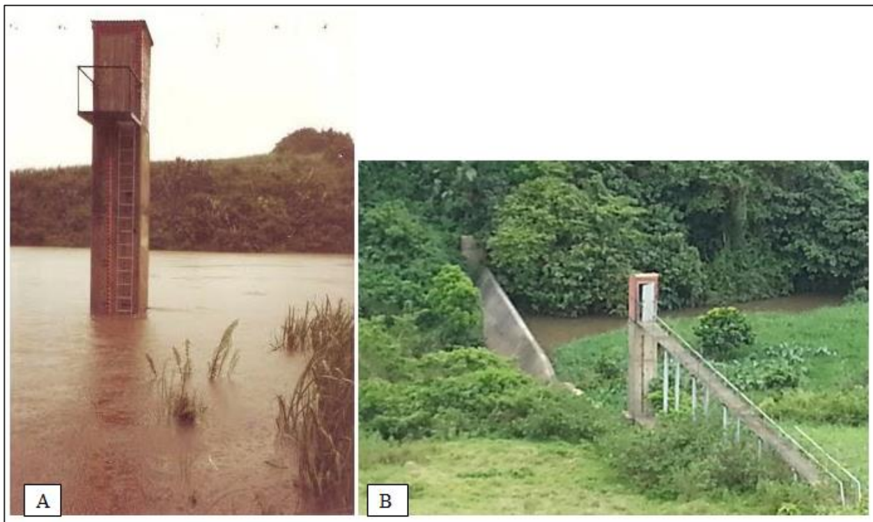
Figure 3.11: W1H012 during 1987 Flood (A) and in 2000 when it was repaired (B) (Photos by B Kelbe)
